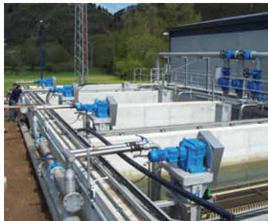
BG Series gear motors are utilized in membrane filtration process.
