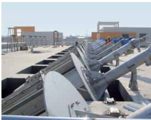
Beijing wastewater pre-cleaning and fine screening operation is powered by Bauer BF Series gear motors.
