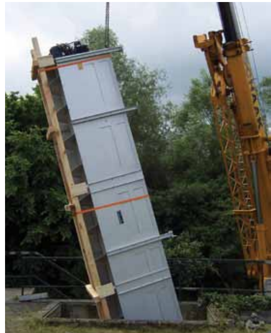
23 metre long screening plant, driven by Bauer BK Series gear motors, is installed in rain overflow basin.
